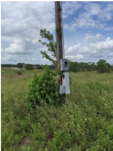
Photo 29 Electrical utilities, Parcel 1.
