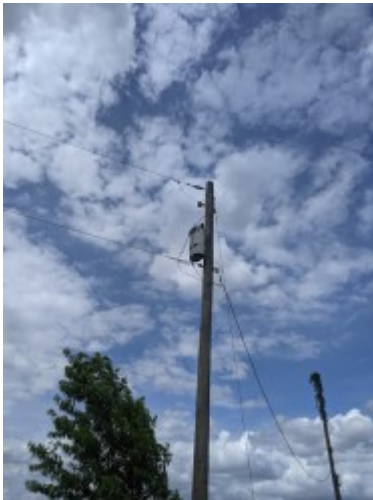
Photo 27 Pole mounted transformer, Parcel 1.
