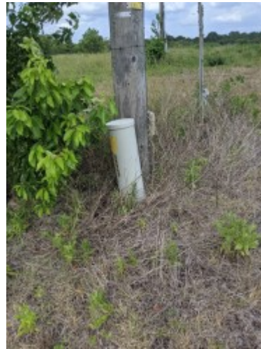
Photo 28 Communications utility connections, Parcel 1
