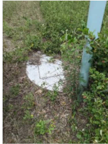
Photo 20 Reuse water line valve manhole, Parcel 2.
